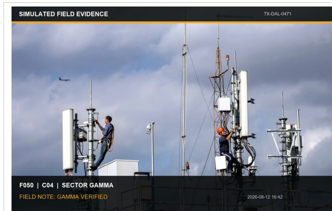
C04 | Gamma: Antenna installation and mounting hardware are visible
